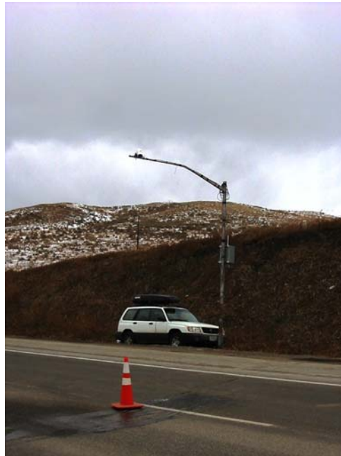
Figure 3-2: IceSight Installed on Mast above RWIS Sensor
