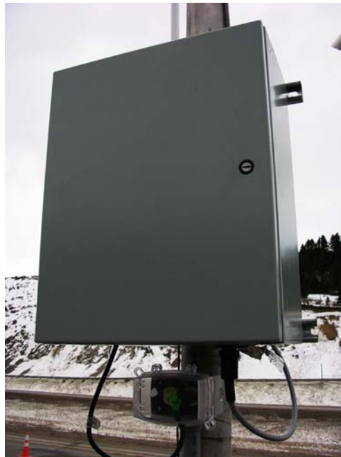
Figure 3-1: IceSight Electrical Supply
