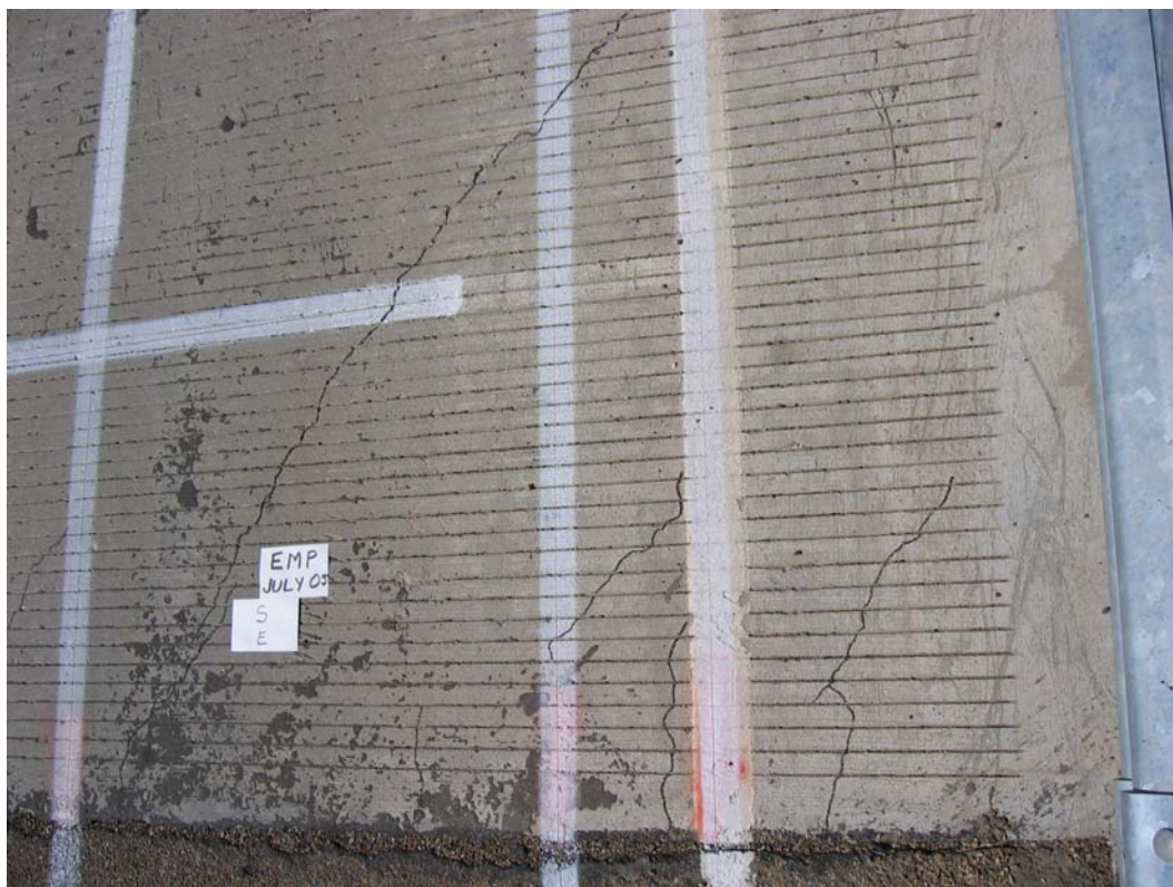
Figure H -15: Top-Surface Cracking at East Side of South Abutment – Empirical Deck
