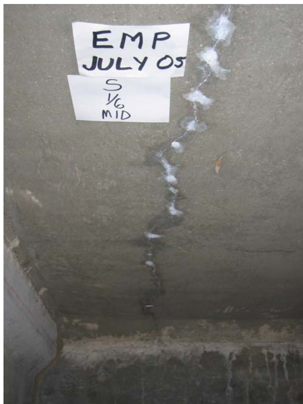
Figure H -20: Full-Depth Crack near Center of South End (shown from underside) – Empirical Deck
