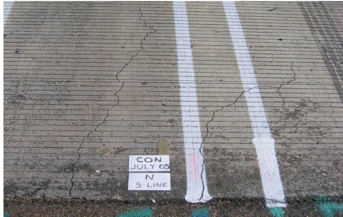
Figure 108: Top-Surface Cracking at West Side of North Abutment – Conventional Deck
