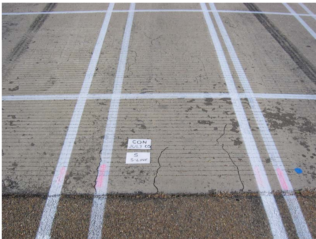
Figure H -6: Top-Surface Cracking at South Abutment – Conventional Deck
