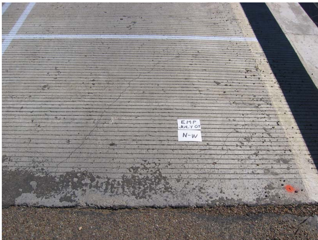
Figure H -14: Top-Surface Cracking at West Side of North Abutment – Empirical Deck
