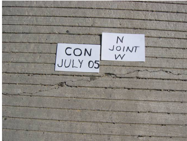
Figure 105: Full-Depth Transverse Crack at Northern-Most Interior Bent – Conventional Deck
