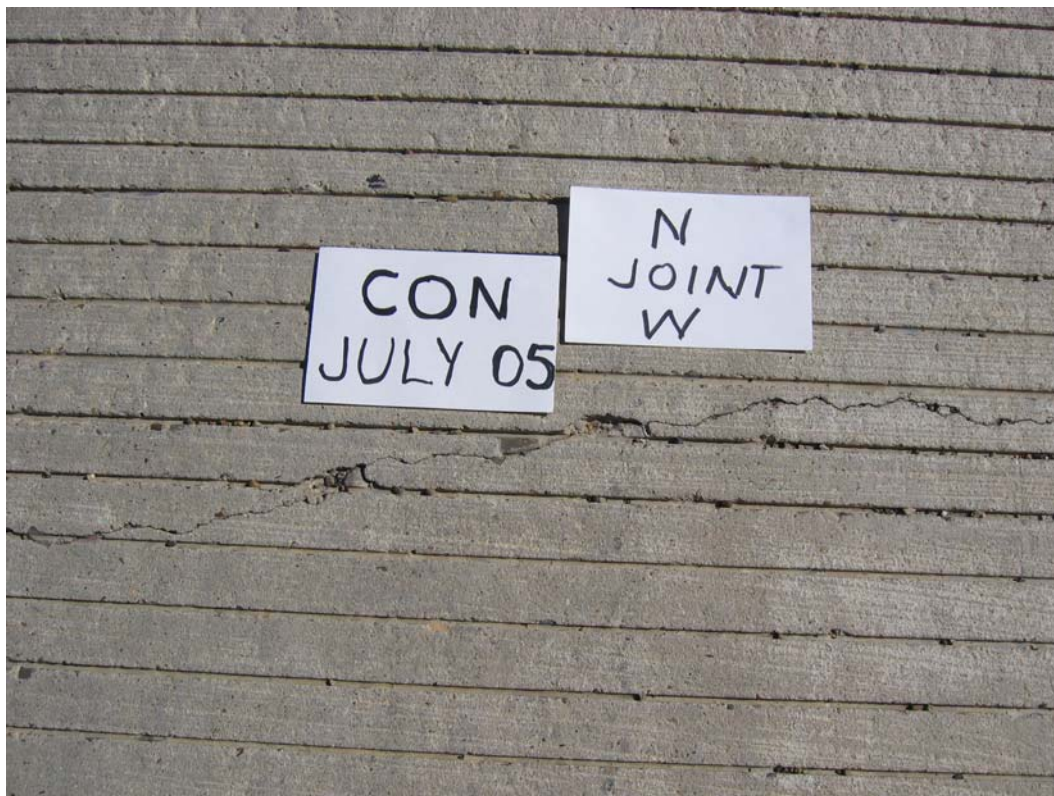
Figure H -3: Full-Depth Transverse Crack at Northern-Most Interior Bent – Conventional Deck
