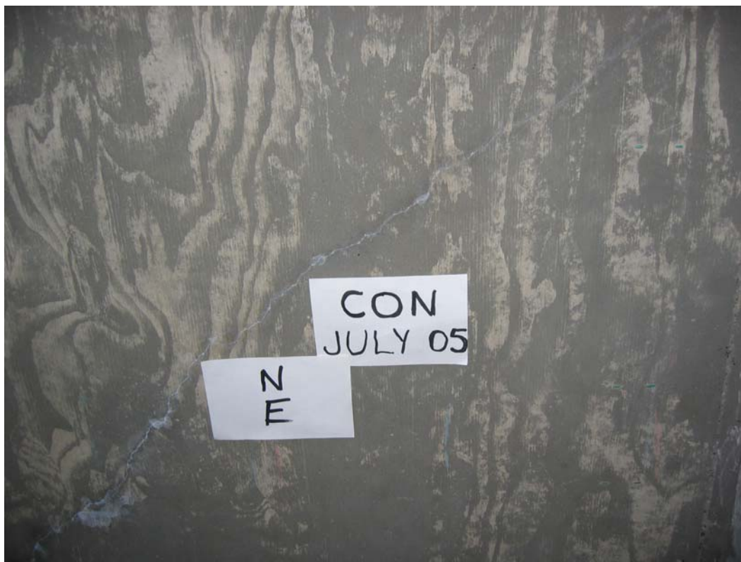
Figure H -7: Full-Depth Crack at Northeast Corner (shown from underside) – Conventional Deck
