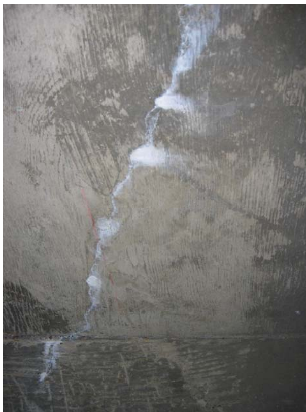
Figure H -19: Full-Depth Crack at Southeast Corner (shown from underside) – Empirical Deck
