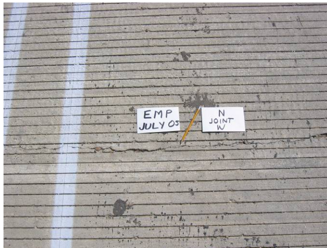
Figure 106: Full-Depth Transverse Crack at Northern-Most Interior Bent – Empirical Deck
