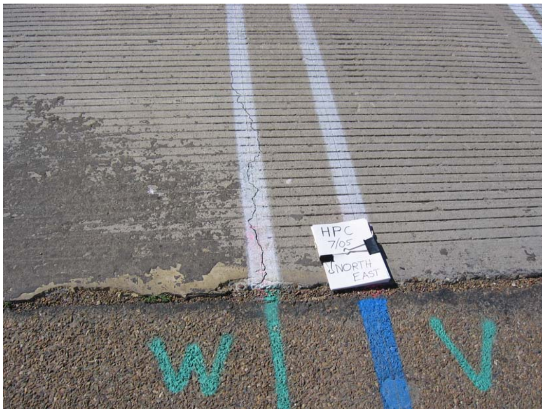
Figure H -29: Top-Surface Cracking at East Side of North Abutment – HPC Deck
