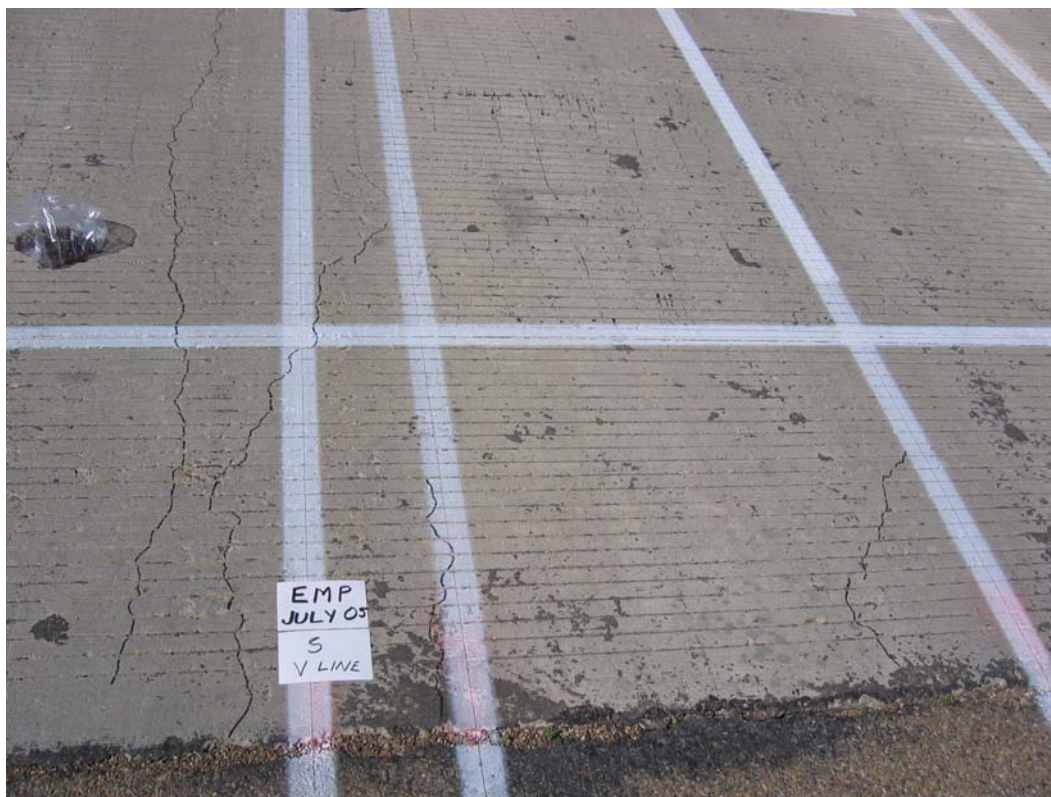
Figure H -16: Top-Surface Cracking at South Abutment – Empirical Deck
