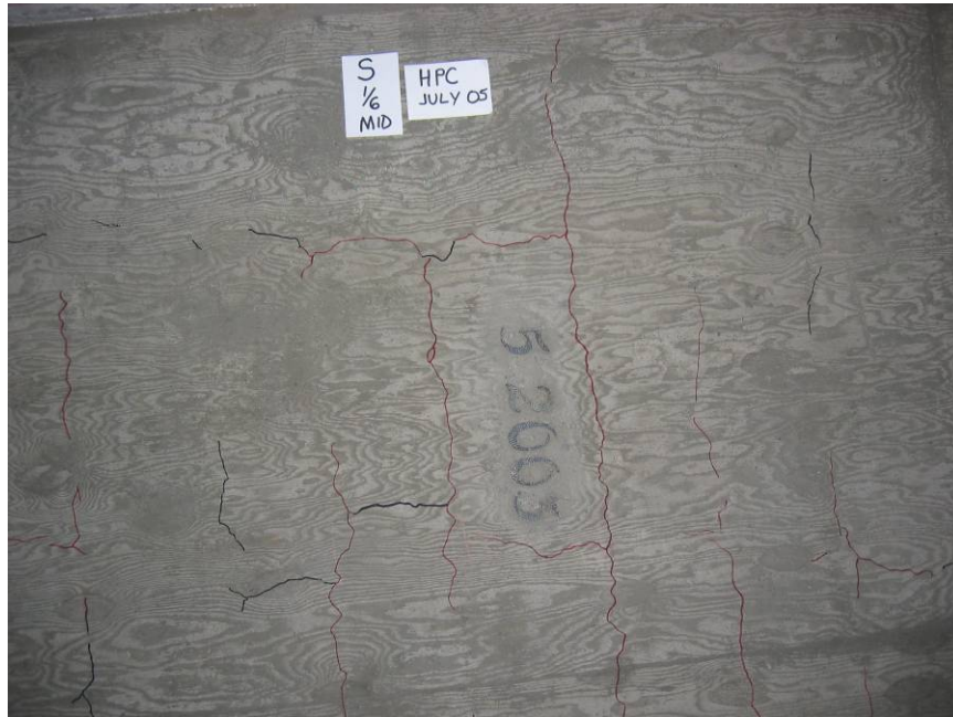
Figure 113: Hairline Cracking near South Abutment (shown from underside) – HPC Deck
