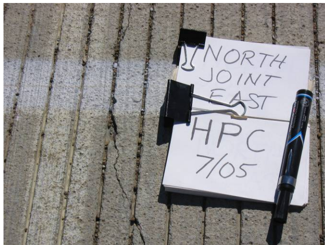
Figure 107: Full-Depth Transverse Crack at Northern-Most Interior Bent – East HPC Deck
