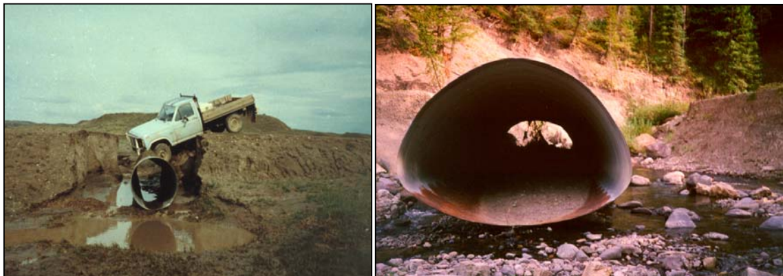
Figure 1. Culverts that failed during extreme flows.
