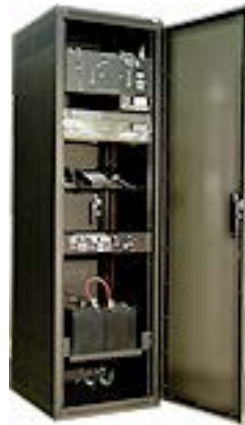
Figure 5: Highway Advisory Radio Station
