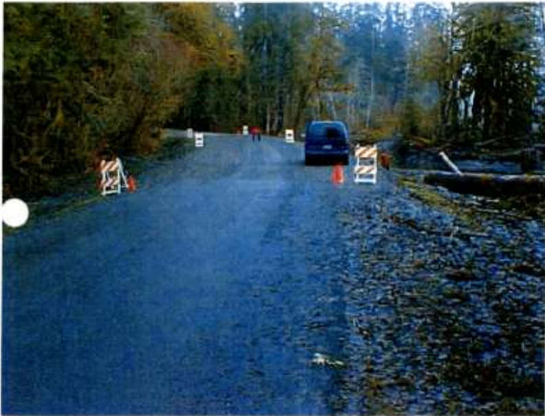
Roadway Washout - emergency/permanent repairs completed (without final surfacing and log crib mitigation)
