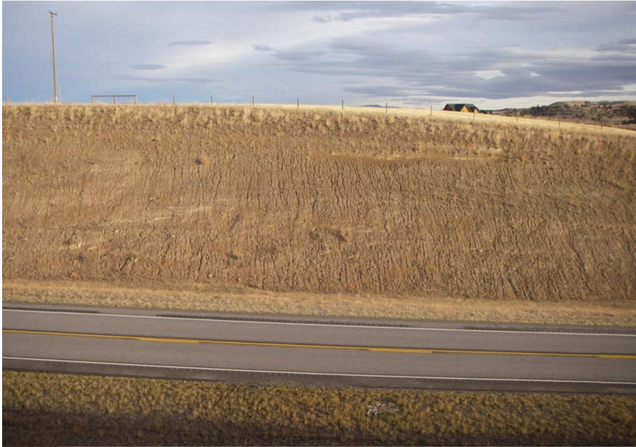
Figure 6: Evidence of erosion and sparse vegetation on the westernmost section of the south-facing cut slope, prior to test plot construction.
