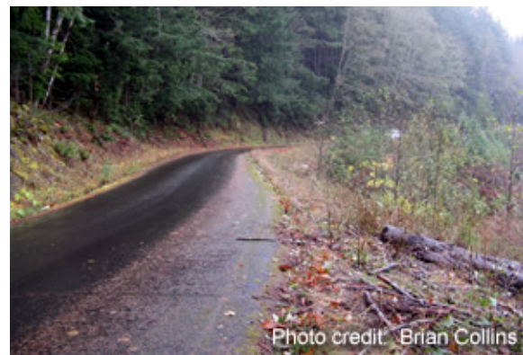
FDR 26 in 2010. Deep patch was applied in 2001.
