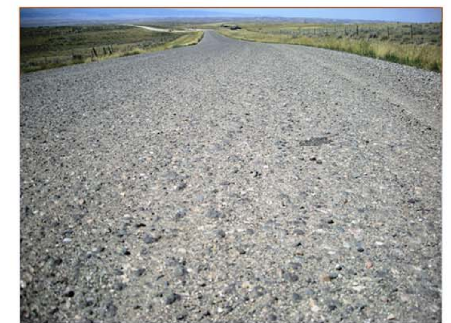
Blended RAP without CaCl three months after placement.
