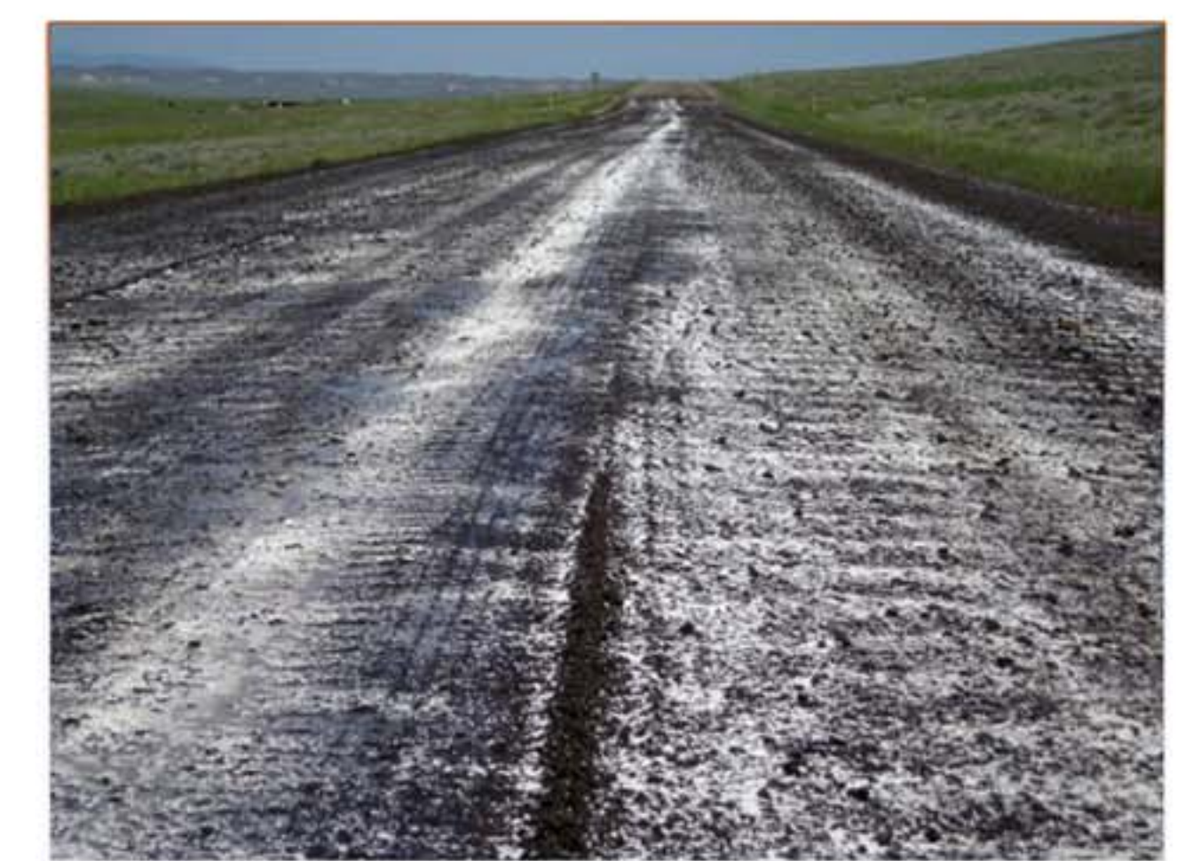
RAP blend sections with and without CaCl flakes. Water was applied, then flakes, then additional water.
