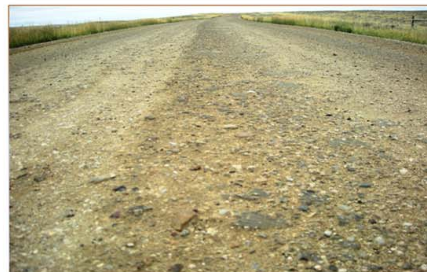
Schoonover Road section S0 aggregate control with CaCl three months after placement
