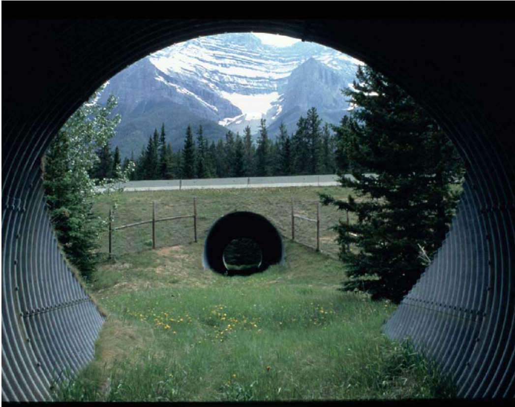
Photo 4. Example of one of twenty-two wildlife underpasses constructed to mitigate the doubling of the busy Trans-Canada Highway.
