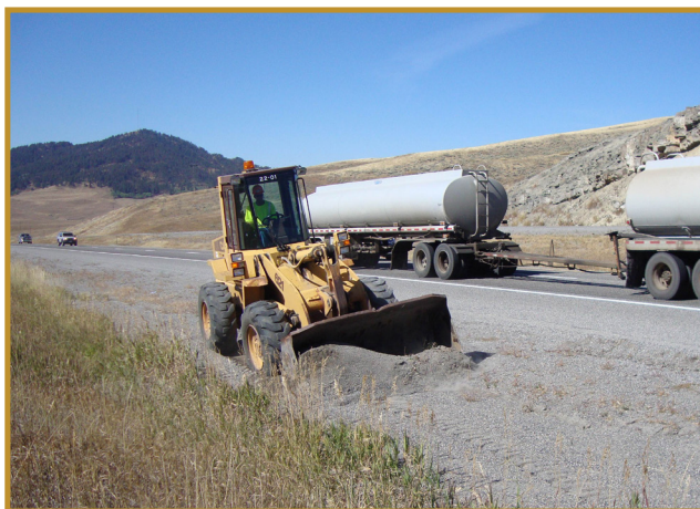
Figure 1 - Cleaning previously deployed traction sand from the roadway shoulder of I 90 near Bozeman Pass
