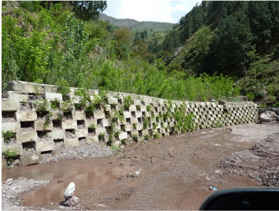
FIGURE 28 POST-EARTHQUAKE (2005) SLOPE STABILIZATION USING A MASONRY CRIB WALL AND LAYERED PLANTING OF NATIVE TREES AND BUSHES, BALAKOT-KAGHAN ROAD (N-15), PAKISTAN. PHOTO PROVIDED BY A. FAIZ.
