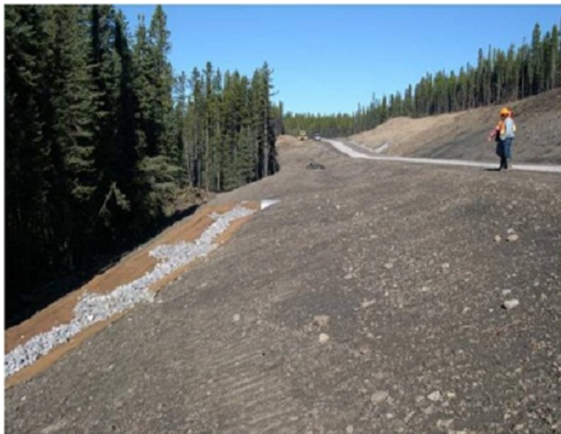
FIGURE 9 GEOTEXTILE- AND ROCK-LINED DITCH EXAMPLE OF SURFACE DRAINAGE. PHOTO PROVIDED BY C. GILLIES.
