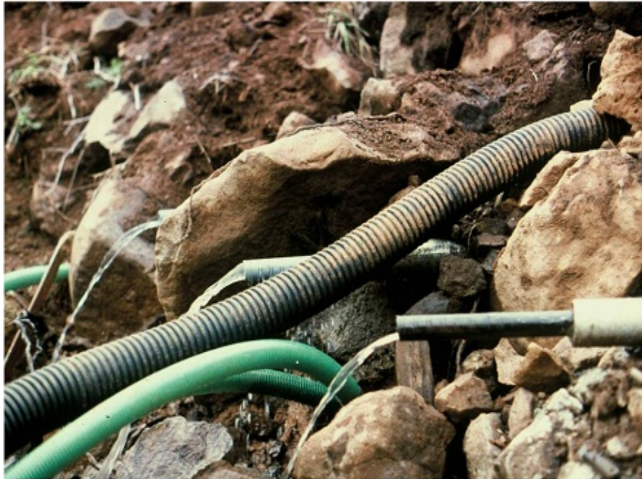
FIGURE 13 OUTLET OF HORIZONTAL SUBSURFACE SLOPE DRAINAGE. PHOTO PROVIDED BY M. LONG.
