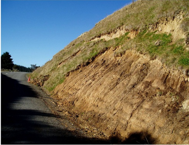
FIGURE 4 SHALLOW CUT FAILURE JUST BELOW GRASS ROOT DEPTH. PHOTO PROVIDED BY G. KELLER.
