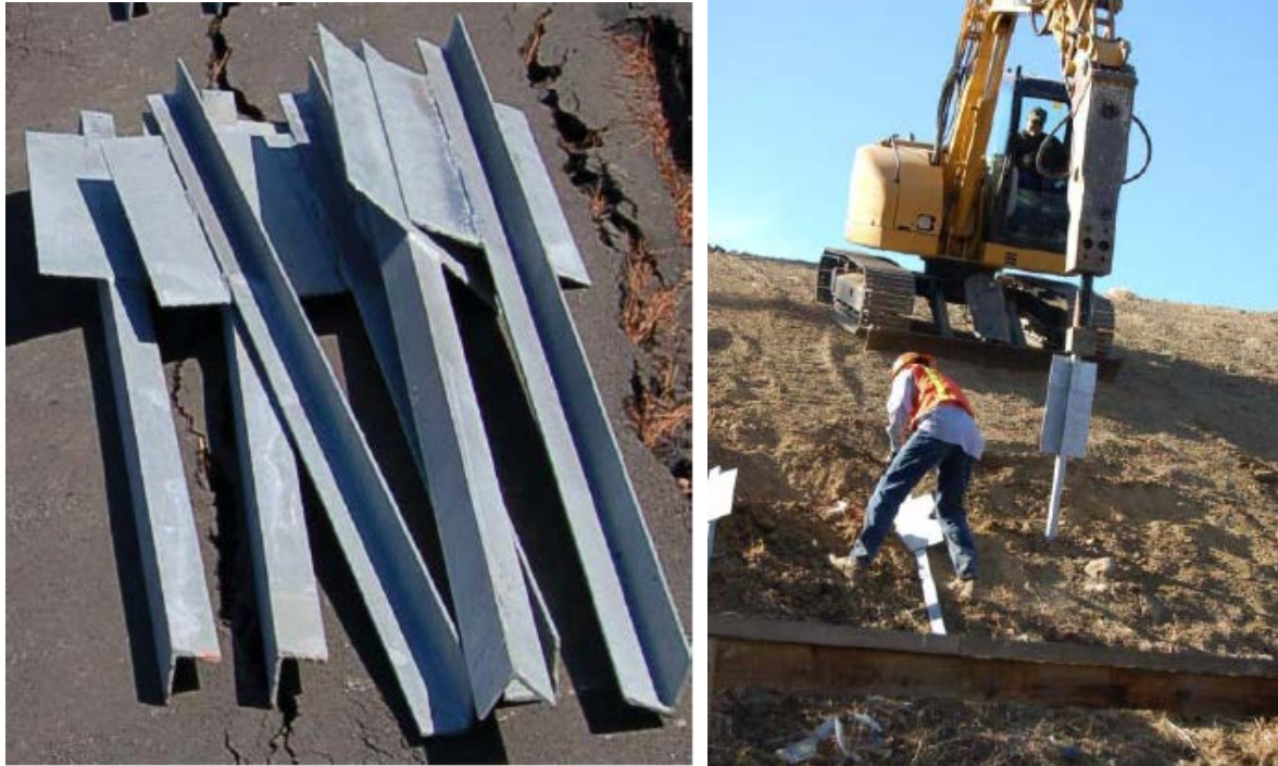
FIGURE 40 6-FOOT PLATE PILES (LEFT) AND PLATE PILE INSTALLATION (RIGHT) USING AN EXCAVATOR WITH A HYDRAULIC HAMMER. PHOTOS PROVIDED BY Y. PRASHAR.
