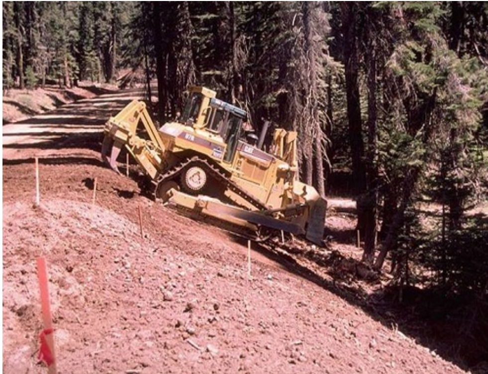
FIGURE 42 ROUGHENED SOIL AND TRACKWALKING WITH HEAVY EQUIPMENT. PHOTO PROVIDED BY G. KELLER
