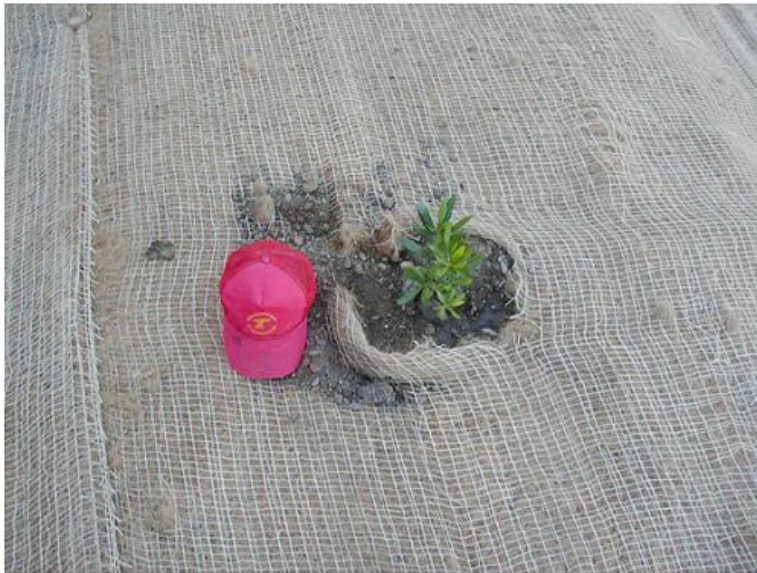
FIGURE 17 BIODEGRADABLE NETTING WITH PLANTED VEGETATION, FLORAS CREEK, OREGON. PHOTO PROVIDED BY M. LONG.
