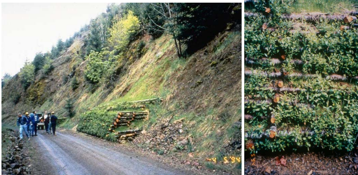
FIGURE 27 LIVE CRIB WALL, FROM A DISTANCE (LEFT) AND CLOSE UP (RIGHT). PHOTOS PROVIDED BY G. KELLER
