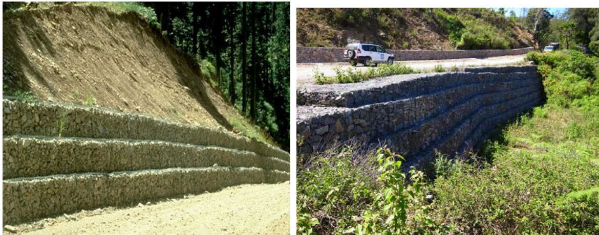
FIGURE 34 LOW GABION WALL AND GABION WALL STABILIZATION AT TOP OF FILL SLOPE IN TIMOR. PHOTOS PROVIDED BY G. KELLER AND C. BENNETT.
