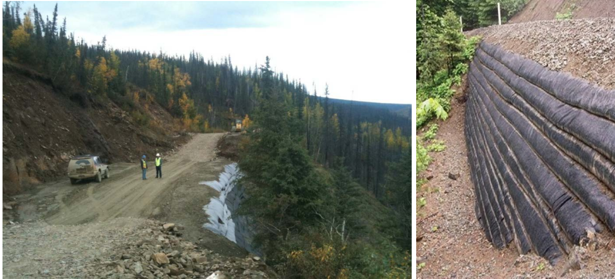
FIGURE 36 EARLY WORK BY A CONTRACTOR CREATING A GEOTEXTILE WALL IN ALASKA, AND GEOTEXTILE WALL ON FILL SLOPE OF ROAD IN KLAMATH NATIONAL FOREST IN CALIFORNIA. PHOTOS PROVIDED BY J. CURREY AND G. KELLER.
