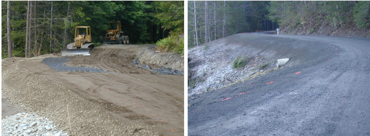
FIGURE 37 DEEP PATCH DURING AND AFTER CONSTRUCTION IN GIFFORD PINCHOT NATIONAL FOREST IN WASHINGTON. PHOTOS PROVIDED BY B. COLLINS.
