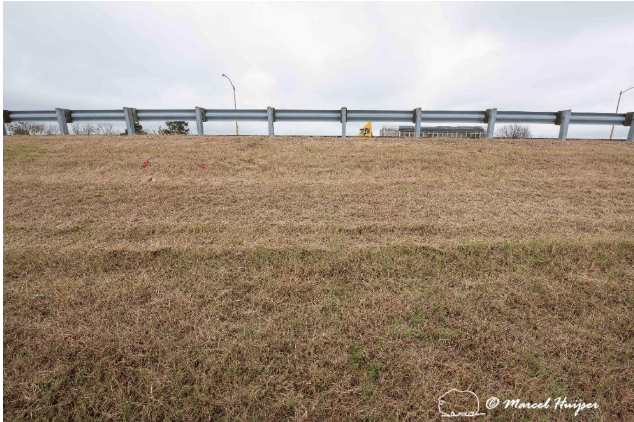
Figure 31: The roadbed, showing the potential for drilling culverts under highway, US Hwy 13, Fisherman Island NWR.
