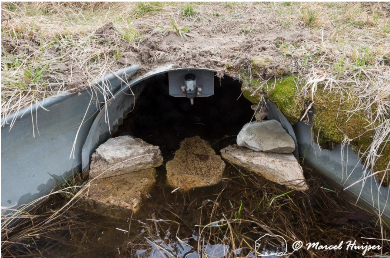
Figure 33: Camera facing down to record turtles, and rock ramp in culvert to force turtles above the water surface when crossing through the culvert, Valentine NWR, Nebraska, USA.
