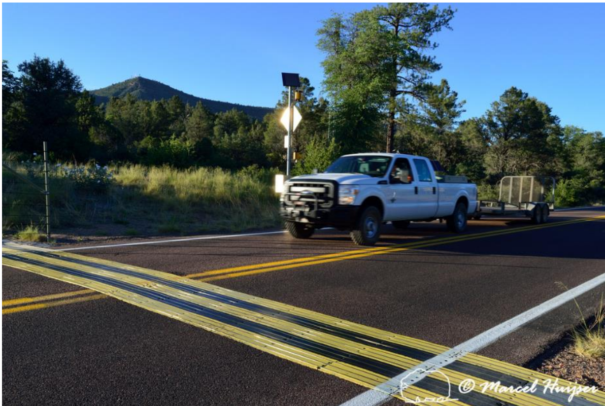
Figure 38: Electric mat (Electrobraided™ / CrossTek™) associated with an animal detection and driver warning system at a fence end, S.R. 260 east of Payson, Arizona, USA.
