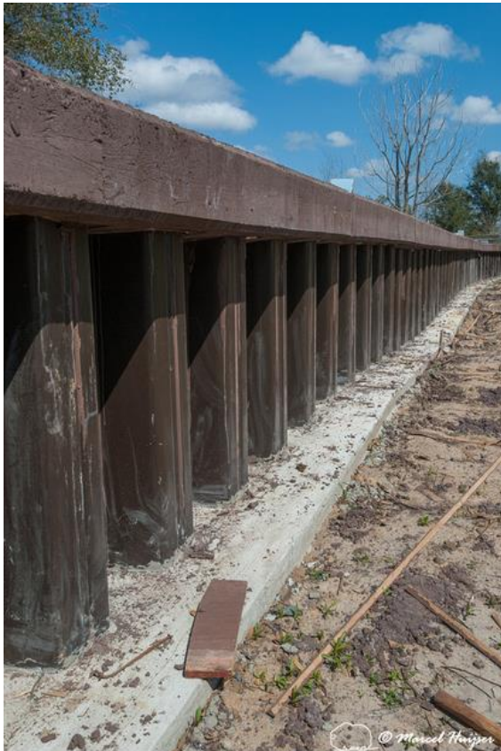
Figure 23: Barrier wall under construction with concrete top and overhang or 'lip', Lake Jackson Ecopassage, U.S. Hwy 27, Tallahassee, Florida, USA. The barrier wall (height 5 ft) is designed for turtles, alligators, snakes and amphibians.
