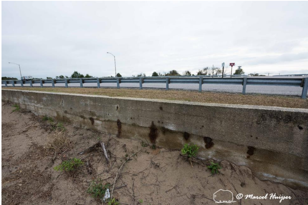
Figure 24: Existing concrete barrier wall along west side U.S. Hwy 13, Fisherman Island National Wildlife Refuge, Virginia, USA.
