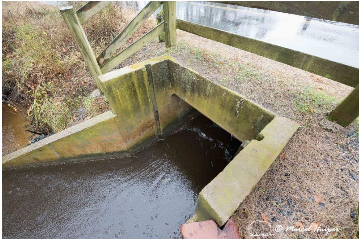
Figure 47: Box culvert at the current beach access road, Chincoteague National Wildlife Refuge, Virginia, USA.
