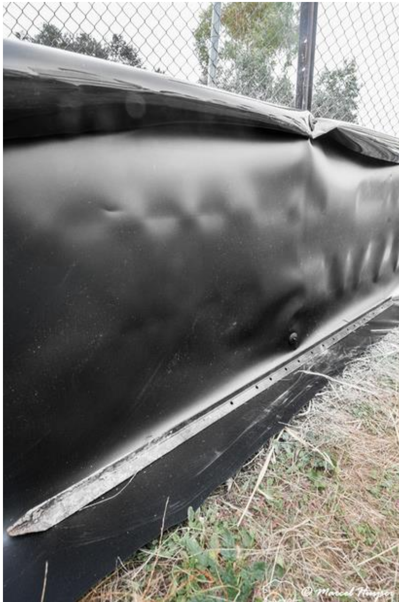
Figure 20: Temporary demonstration installation of solid smooth plastic fence sheets (high-density polyethylene, Animex) designed as a barrier for herpetofauna, near Ballarat, Victoria, Australia.
