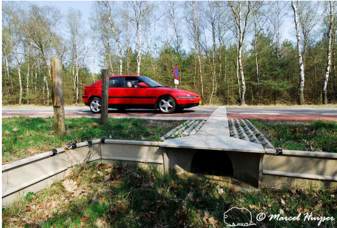
Figure 29: Example of an amphibian barrier wall and a dry amphibian tunnel (ACO) with an open slotted roof embedded in the pavement under a 2-lane road, Deelenseweg, between Hoenderloo and Arnhem, Gelderland, The Netherlands.
