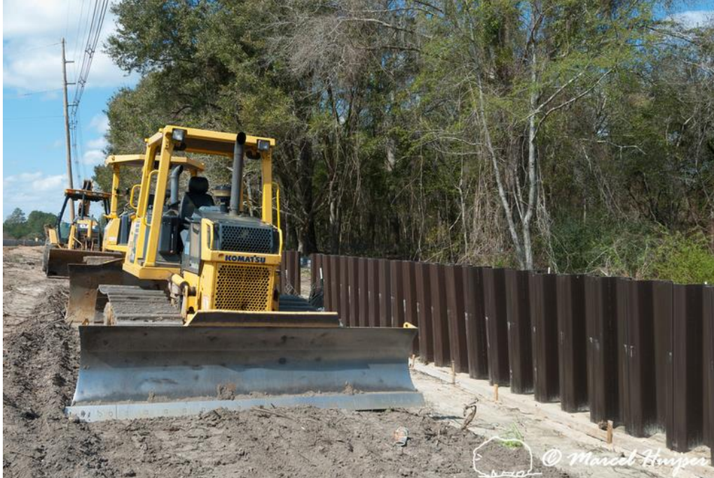
Figure 22: Barrier wall under construction, Lake Jackson Ecopassage, U.S. Hwy 27, Tallahassee, Florida, USA. The barrier wall (height 5 ft) is designed for turtles, alligators, snakes and amphibians.
