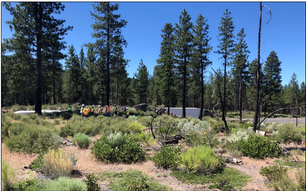
Figure 54: Grass Lake B looking south towards US-97 showing the little fill required for the approach ramps.
