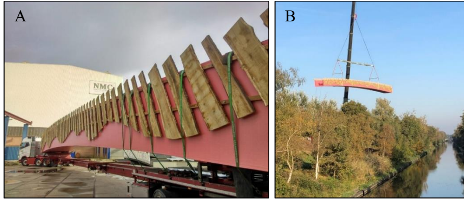
Figure 10: A) FRP uni-mold bridge is delivered in one piece from the factory to the construction site; B) bridge is installed using one crane (FiberCore Europe, 2019b).
