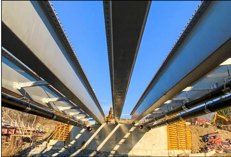
Figure 36: The CT girder bridge system installed during first construction in Hampden, Maine, 2020 (Advanced Infrastructure Technologies, 2020).
