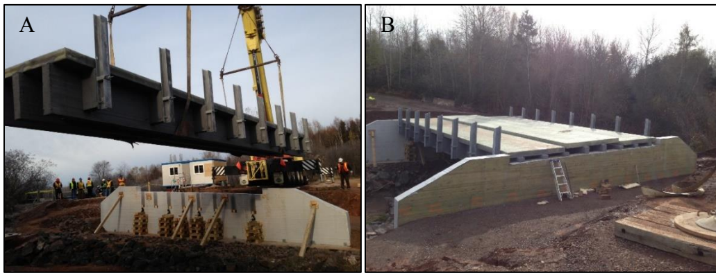
Figure 17: Wood and FRP bridge made by Guardian Bridge Rapid Construction for a two-lane road; A) a triple-tee span being placed by a crane; B) all three spans placed on top of an FRP abutment.
