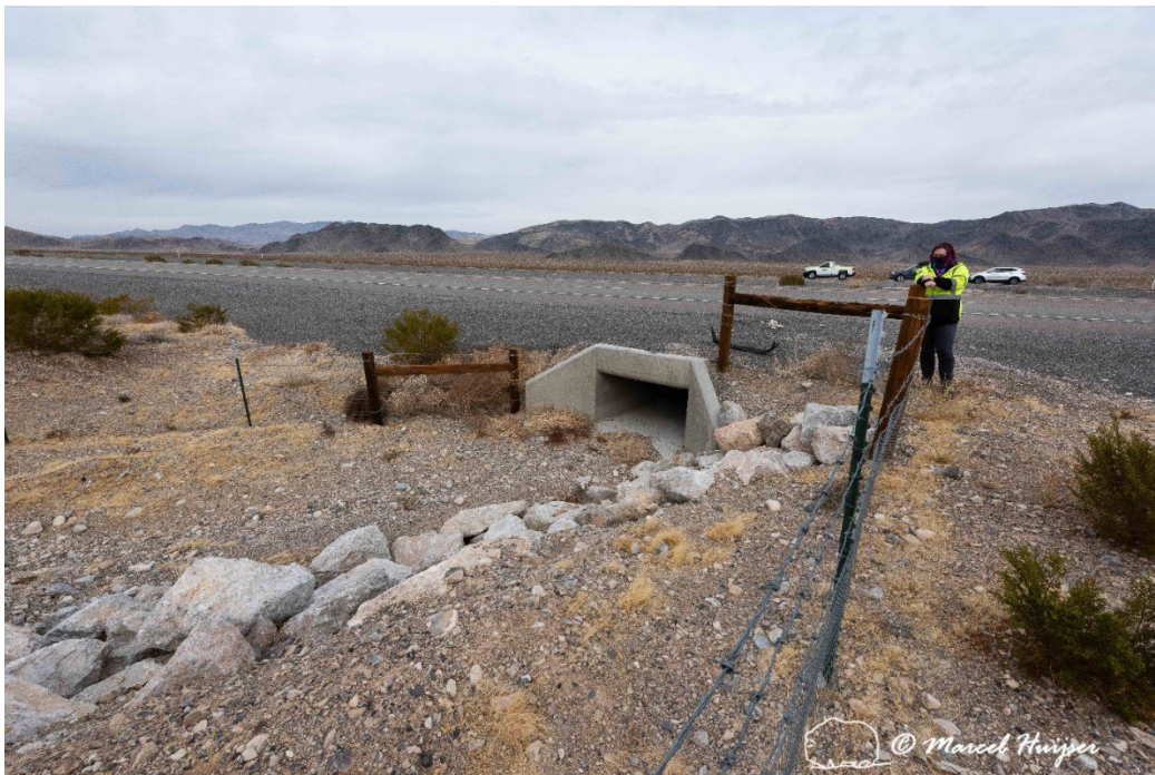
Mojave desert tortoise fence and a culvert US Hwy 95 (MP 127.5 SB) near Indian Springs, Nevada. Riprap stabilizes the slope between the fence and the culvert. Mojave desert tortoises that follow the fence cannot easily access the culvert; they would have to navigate the riprap on the slope first. Design and construction of culverts, fences, and measures aimed at erosion control should ensure that tortoises can easily access the culvert, including when they follow the fence.
