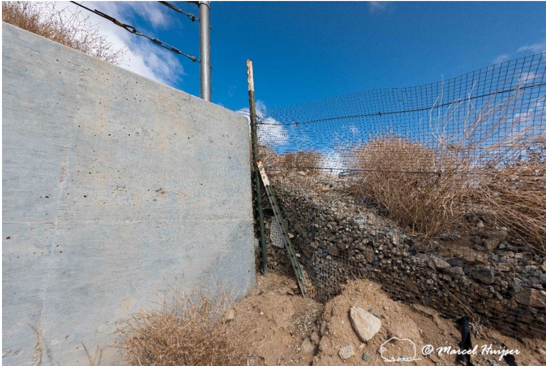
Mojave desert tortoise fencing connected to a culvert, I-15 near Barstow, California. Here debris (rocks, sand) has built up against the fence, threatening its integrity.
