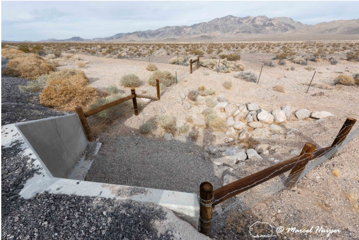
Mojave desert tortoise fencing connected to a concrete box culvert (lower left), US Hwy 95 (MP 125 NB) near Indian Springs, Nevada. Note that the fences angle from the property boundary towards the culvert to funnel the animals towards the culvert. Also note that the property boundary fence continues through the wash (this property boundary fence is not a barrier to Mojave desert tortoises).
