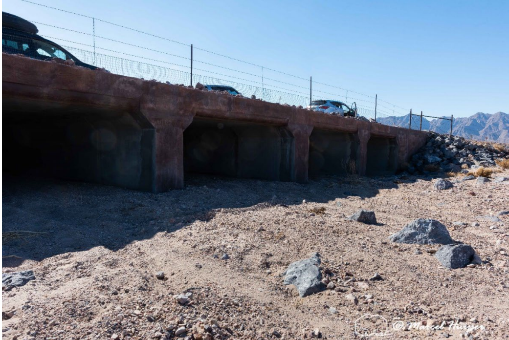
Riprap filled in with finer rocks and sand, in front of culverts to reduce erosion, I-11, near Boulder City, Nevada. This does not appear to be a barrier to Mojave desert tortoises.
