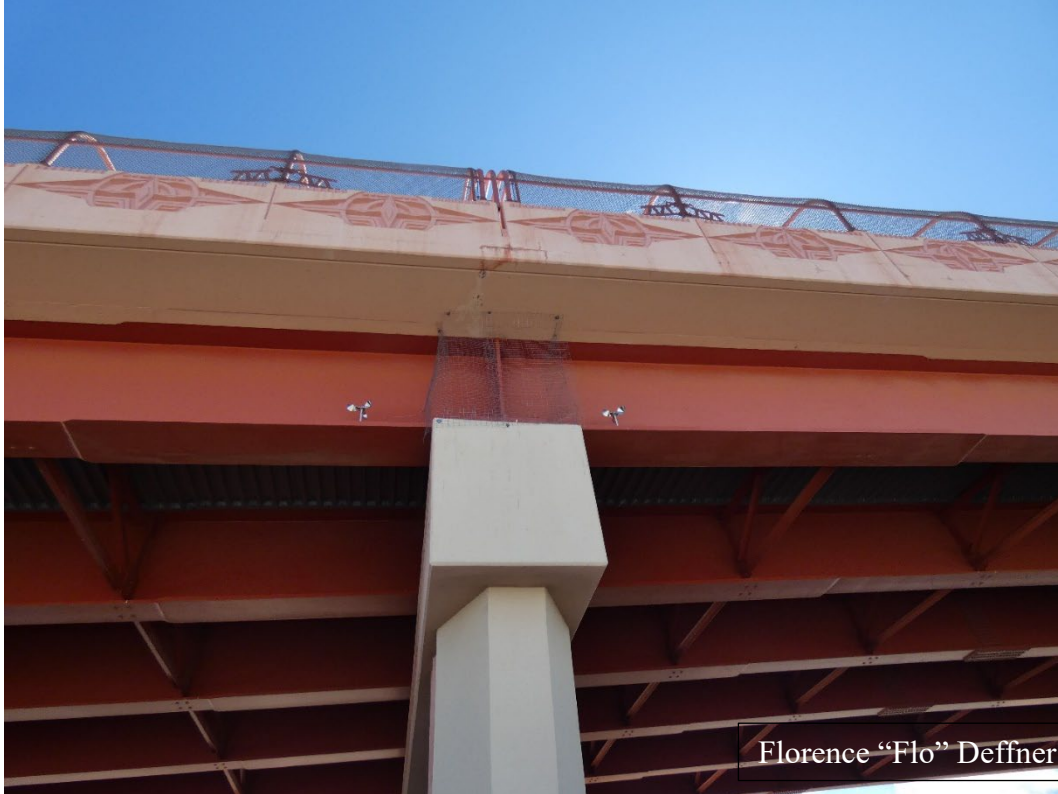
Wire mesh and metallic flashers installed to discourage raven nesting on Snow Mountain Overpass, U.S. 95, Las Vegas, Nevada.
