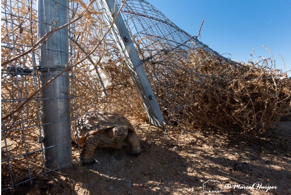
Gap at a gate associated with Mojave desert tortoise exclusion fencing, Hwy 58 near Kramer Junction, California. The gate does not have a buried component, and it had enough flex to result in permanent openings, partially as a result of tumbleweeds being blown against the fence.
