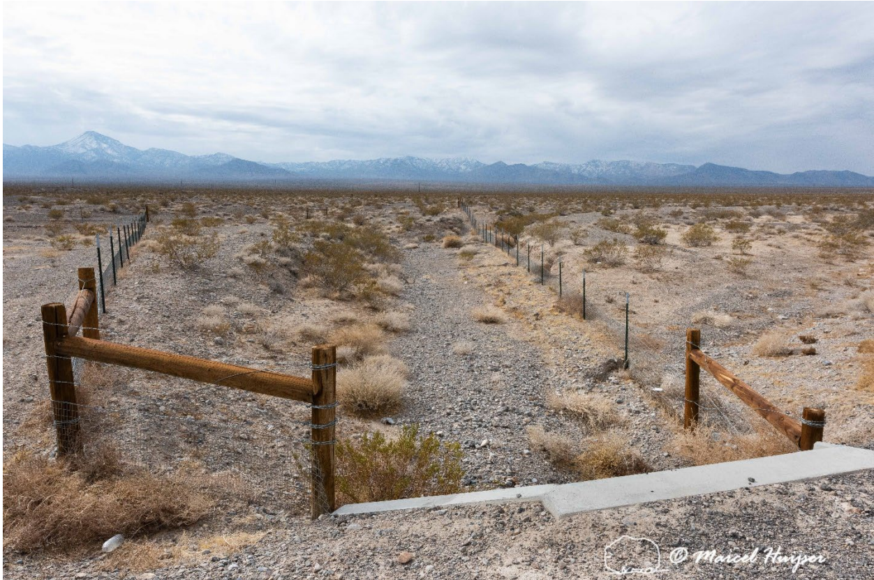
Funnel fencing for Mojave desert tortoise and a box culvert (foreground), US Hwy 95 (MP 126.5 SB) near Indian Springs, Nevada. Note that the fence on the left is on higher ground, on top of the bank of the wash, and not within the wash or on the bank.
