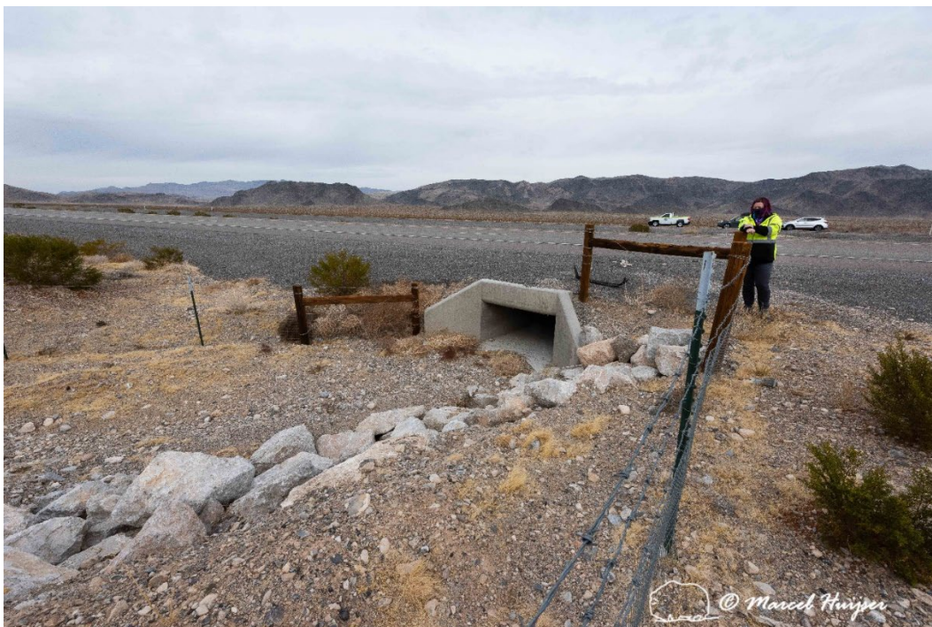
Mojave desert tortoise fencing and a concrete box culvert, US Hwy 95 (MP 127.5 SB) near Indian Springs, Nevada. Note that the fence on the near side is located on top of the bank of the desert wash, and not in the wash or on the bank.
