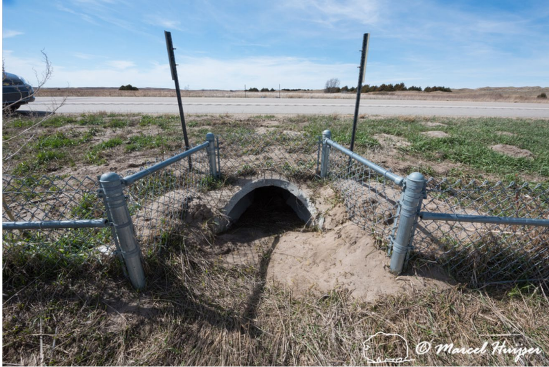
Turtle fence and a dry culvert used by turtles, Valentine National Wildlife Refuge, Ballard's South, Valentine, Nebraska, USA. This culvert is 30 inches wide, 22 inches tall. Note that this turtle fence has no gap and continues behind and on top of the culvert.
