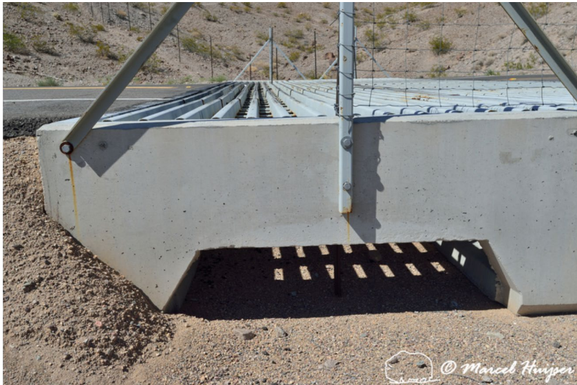
Combined drainage and escape for small animal species under a wildlife guard, Arizona, USA. While the metal bar design of this particular wildlife guard is not appropriate as a barrier for Mojave desert tortoises, the openings on the concrete walls on the side allow invertebrates, amphibians, reptiles, small mammals and other species that may fall in between the metal bars to escape to the safe side of the fence (not the roadside). For wildlife guards that have a fully enclosed pit with contiguous walls wooden planks or metal strips are sometimes attached, allowing animals to climb out of the pit. Wildlife guards are no longer recommended because Mojave desert tortoises may still cross and there may be maintenance issues if debris (e.g., tumbleweed) gets stuck in the pit (Pers. com. Kerry Holcomb, USFWS).
