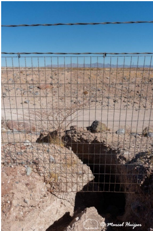
Mojave desert tortoise fencing with soil erosion, I-11, near Boulder City, Nevada. Note that the animals may now move in the erosion gully under the fence. Also note that the fence appears to have only been dug 6 inches into the ground rather than the recommended minimum 12 inches.
