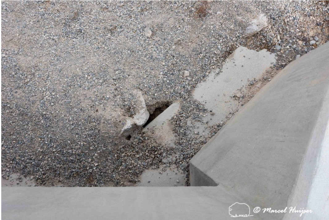
Erosion along a concrete pathway leading up to a concrete box culvert, US Hwy 95 (MP 127.5 NB) near Indian Springs, Nevada. The riprap is filled with finer sediments that allows Mojave desert tortoises to access the culvert. However, it appears that the finer sediments are washing out and resulting in cavities that could trap Mojave desert tortoises.
