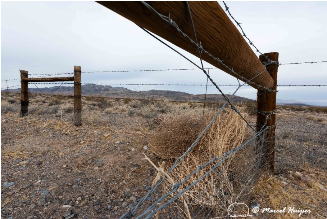
Mojave desert tortoise fence blocking access to a culvert that is considered a danger (e.g., entrapment between riprap or drowning in a deep plunge pool), US Hwy 95 (MP 125 NB) near Indian Springs, Nevada. The decision to block tortoises from accessing the culvert implies that the danger associated with accessing and using a culvert is considered greater than the benefits of potential crossings.
