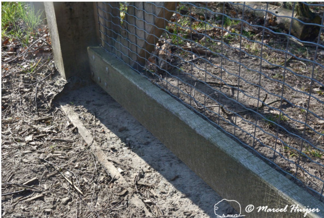
Snug fit of a gate at a wildlife fence, south of Otterlo, The Netherlands. The snug fit discourages animals from crawling under the gate.
