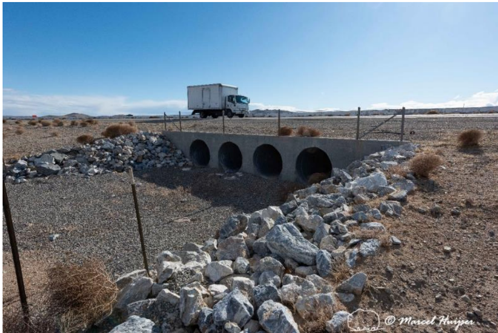
Mojave desert tortoise fencing leading up to culverts primarily designed for hydrology, I-15 near Barstow, California. Note that the fence does not physically connect to the structure and that riprap (rocks) fills the gap. However, it would have been better to leave no gap in the fence and have the fence continue on top of the bank above the boulders.
