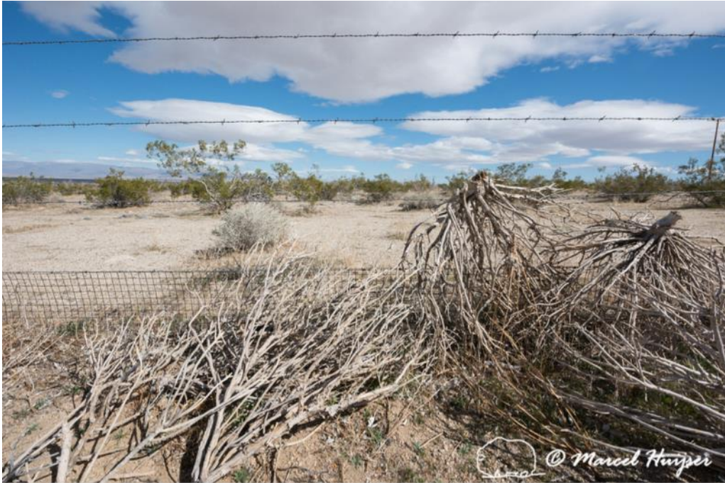
Dead vegetation has blown against the Mojave desert tortoise fence, reducing the barrier effect of the fence to keep tortoise from accessing the highway, Aerospace Hwy, Hwy 14 near Inyokern, California. Note that the height of the fence, as installed, is insufficient to begin with.
