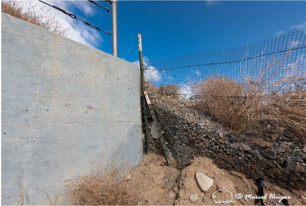
Mojave desert tortoise fencing connected to a culvert, I-15 near Barstow, California. Here debris (rocks, sand) has built up against the fence, threatening its integrity.
