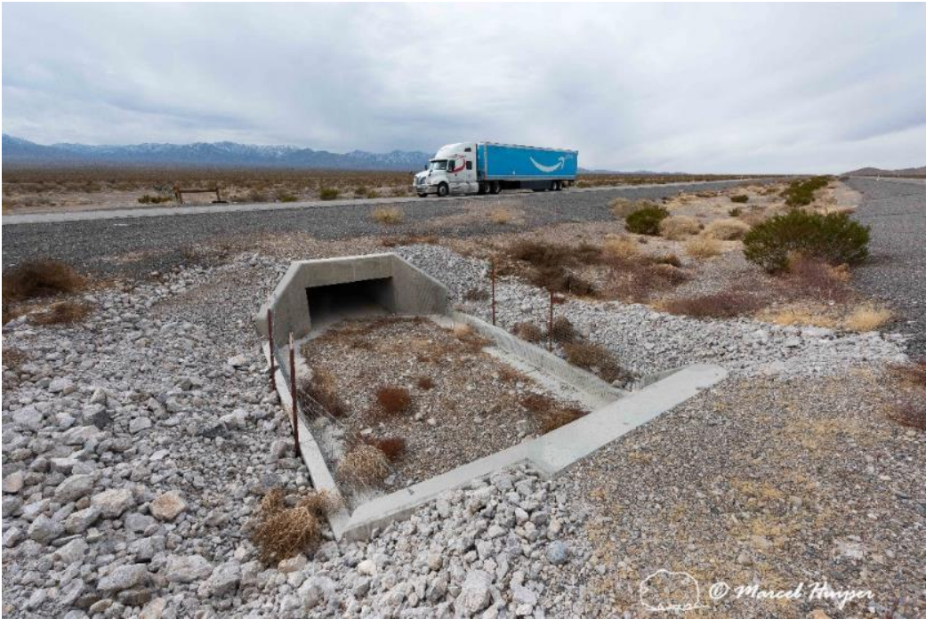
Open medians with separate crossing structures for the two travel directions should have Mojave desert tortoise fencing installed to prevent tortoises from accessing the fenced road corridor in the median.
