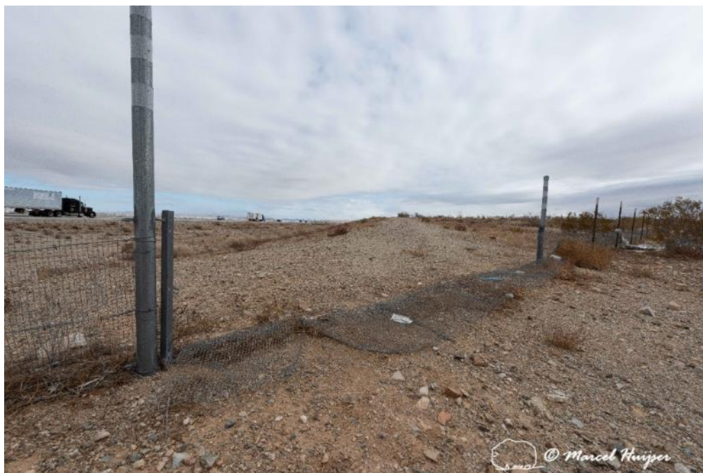
Flattened and destroyed gate at a vehicle access point associated with a Mojave desert tortoise fence, I-15 near Barstow, California. Here the fence has, or had, a gate for a dirt road, but the fence was flattened by vehicles. This suggests that gates that require people to get out of the vehicles to open
