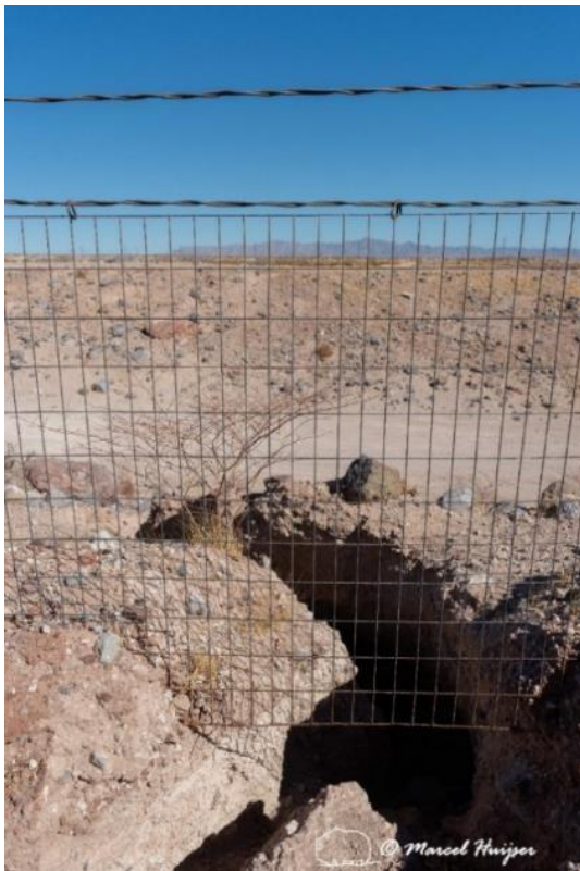
Mojave desert tortoise fencing with soil erosion, I-11, near Boulder City, Nevada. Note that the animals may now move in the erosion gully under the fence. Also note that the fence appears to have only been dug 6 inches into the ground rather than the recommended minimum 12 inches.
