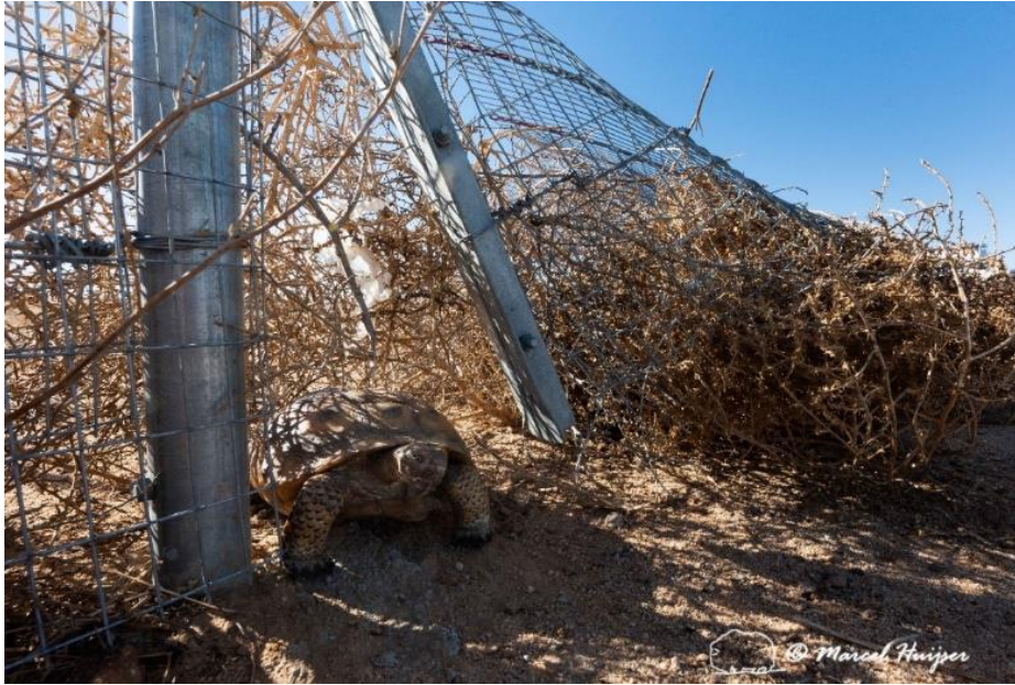
Gap at a gate associated with Mojave desert tortoise exclusion fencing, Hwy 58 near Kramer Junction, California. The gate does not have a buried component, and it had enough flex to result in permanent openings, partially as a result of tumbleweeds being blown against the fence.
