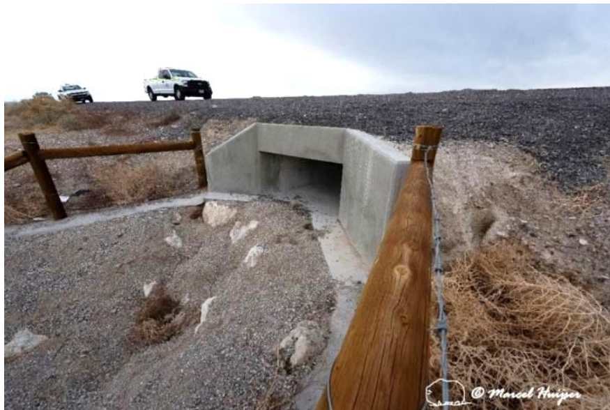
Mojave desert tortoise fence connected to a culvert with concrete pathways leading up to the entrance, US Hwy 95 (MP 121.6 NB) near Indian Springs, Nevada. A deep plunge pool was constructed to address the high water volume and velocity at this outflow. This resulted in substantial erosion and a steep slope, somewhat stabilized by large riprap. The riprap was filled in with smaller substrate to minimize the threat of entrapment of tortoise within gaps formed by the riprap. Concrete pathways were constructed to allow potential use by Mojave desert tortoises for accessing the culvert. The pathways may not be wide enough to allow larger tortoises to turn around with the risk of falling into the plunge pool and erosion is currently undermining the integrity of these pathways. Therefore, this type of culvert access design is not recommended for tortoises.
