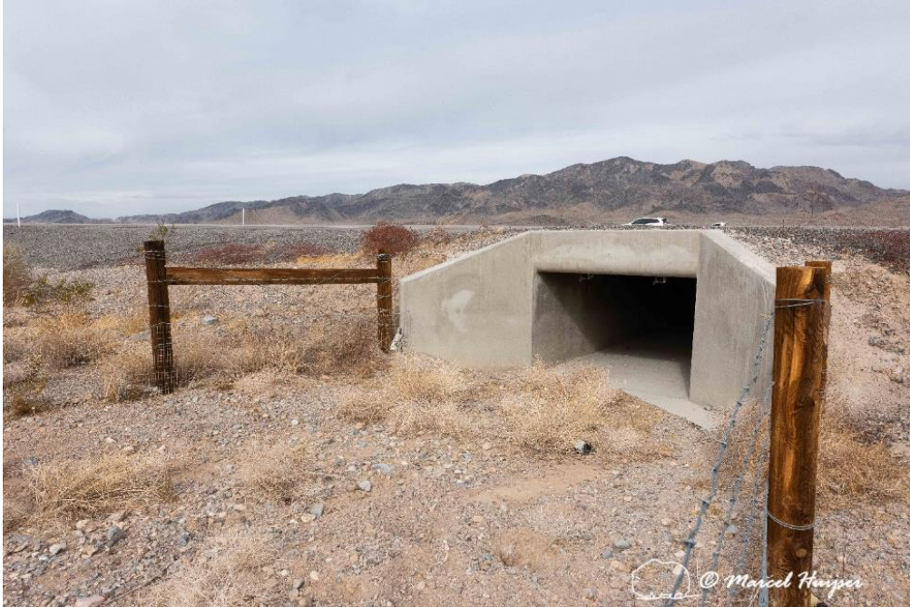
A multifunctional concrete culvert with natural substrate leading up to it, primarily designed for hydrology, but adapted for use by Mojave desert tortoises, US Hwy 95 (MP 125 SB) near Indian Springs, Nevada.
