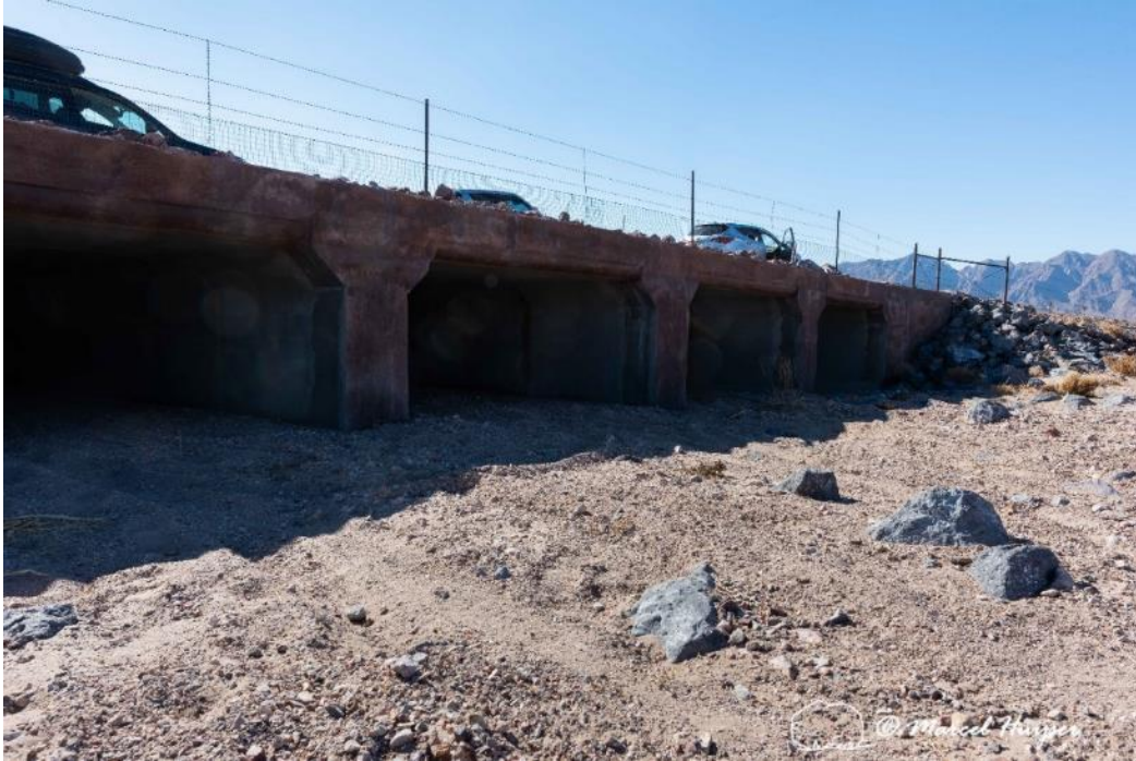
Riprap filled in with finer rocks and sand, in front of culverts to reduce erosion, I-11, near Boulder City, Nevada. This does not appear to be a barrier to Mojave desert tortoises.
