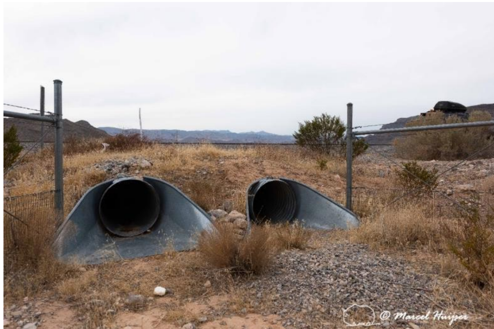
Mojave desert tortoise fencing connected to twin culverts, US Hwy 93 (MP 69.5 NB) near Overton, Nevada. The fencing would be a more effective barrier if it was continued above the culvert without any gap in the fence.
