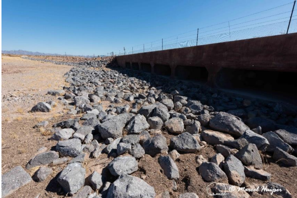
Riprap in front of culverts to reduce erosion, I-11, near Boulder City, Nevada. While beneficial to combatting erosion and sedimentation issues, the size and placement of the riprap most likely results in a substantial barrier to Mojave desert tortoises.
