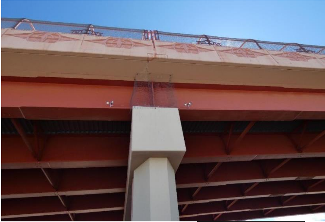
Wire mesh and metallic flashers installed to discourage raven nesting on Snow Mountain Overpass, U.S. 95, Las Vegas, Nevada.
