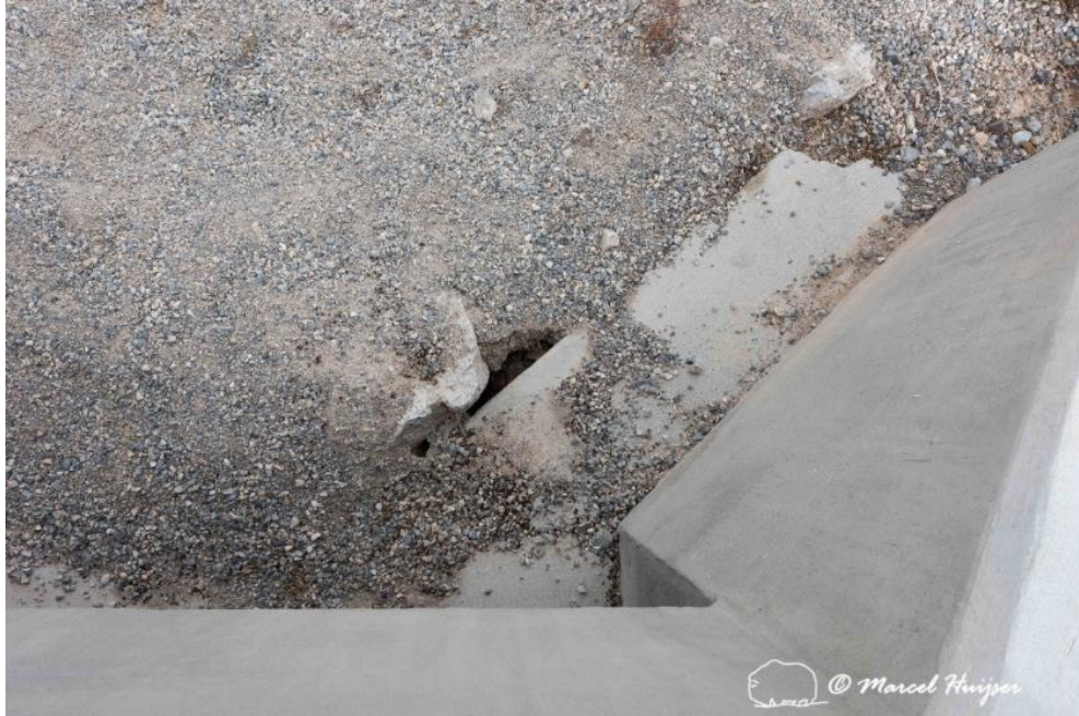
Erosion along a concrete pathway leading up to a concrete box culvert, US Hwy 95 (MP 127.5 NB) near Indian Springs, Nevada. The riprap is filled with finer sediments that allows Mojave desert tortoises to access the culvert. However, it appears that the finer sediments are washing out and resulting in cavities that could trap Mojave desert tortoises.
