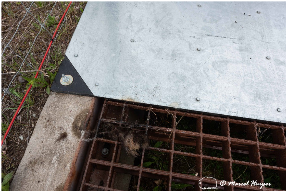
Figure 5: The electrified mat by BS Fabrications covers the concrete edge around the pit, at the north wildlife guard, US Hwy 93, south of Ravalli, Montana.
