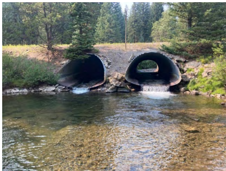
Figure 18 Double Culverts Facilitating Water Flow from Teepee Creek
