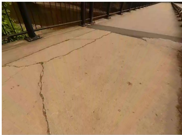
Figure 13: Heavy cracking on concrete trail surface.
