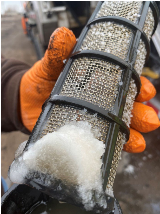
Figure 6. Screen filter clogged with salt crystals.
