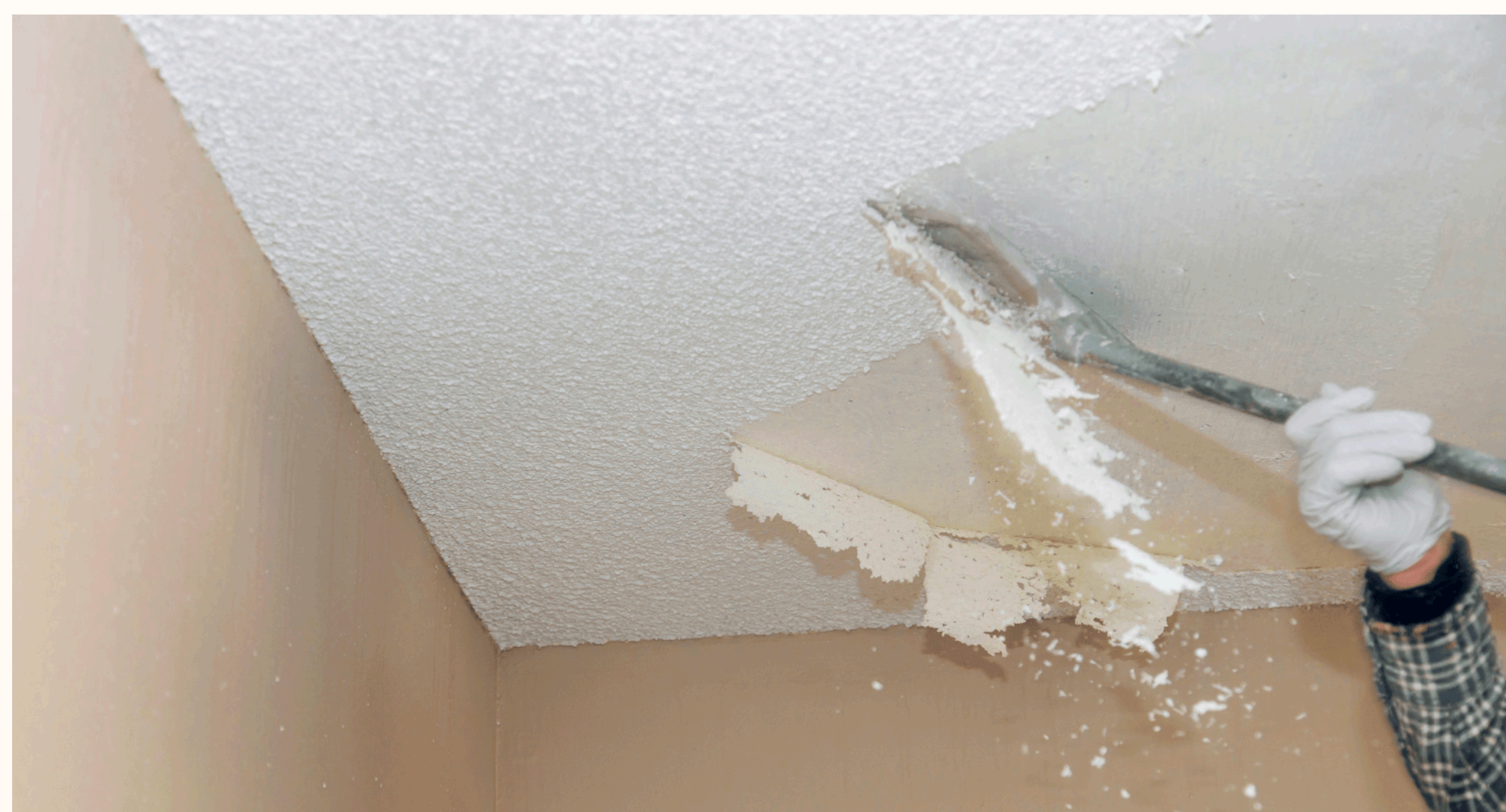
Unsafe removal of a popcorn ceiling containing asbestos Via Homelight.org
