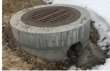
Figure 7: Probable Rating: Fair (2) Large obstruction near opening
