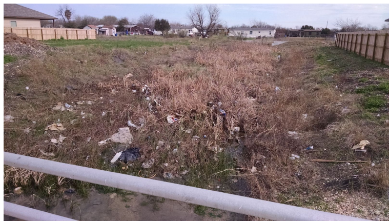
Figure 12: Probable Rating: Poor (3) Overgrown vegetation prevents drainage
