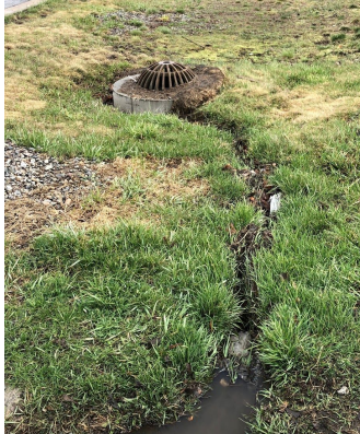
Figure 6: Probable Rating: Poor (3) Erosion around outlet structure
