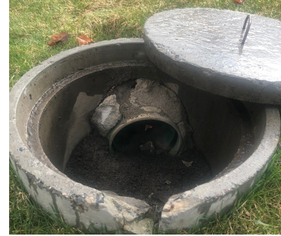
Figure 8: Probable Rating: Fair (2) Sediment build up in basin, structure degrading
