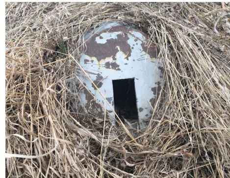
Figure 5: Probable Rating: Poor (3) Surrounding vegetation would likely impede pond function
