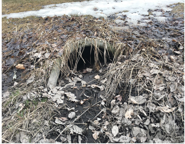
Figure 2: Probable Rating: Extreme (11) Sediment buildup over 66%
