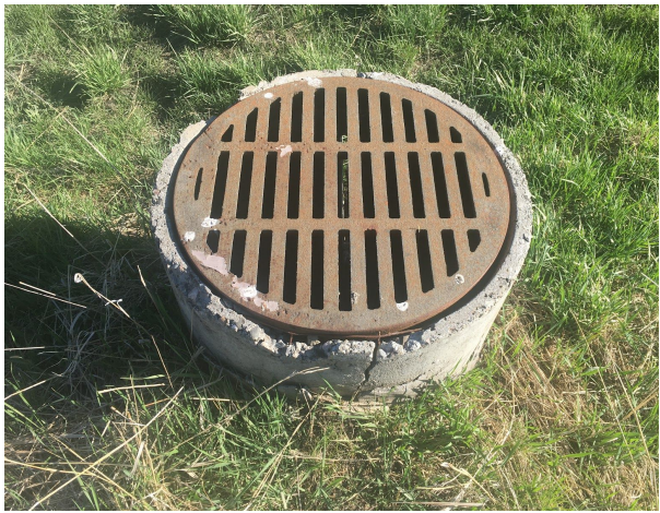
Figure 13: An outlet structure in poor condition. Significant cracking and rebar showing.
