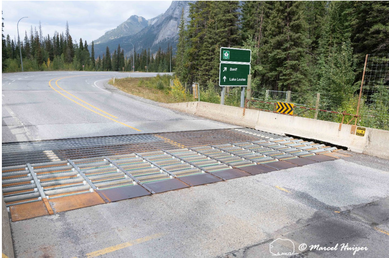
Figure 1: Electrified barrier, Sunshine Road, Banff National Park, Canada
