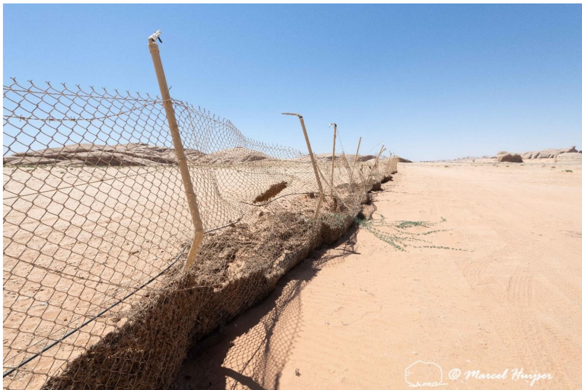
Figure 20: Surface flow and sedimentation damaged the wildlife fence around Sharaan, along Hwy 8806, Alula, Medina Province, Saudi Arabia.
