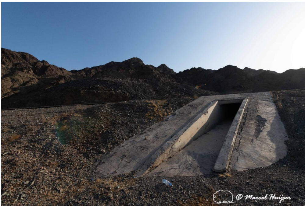
Figure 19: Culvert just north (upstream) from the potential mitigation site for Nubian ibex ( Capra nubiana ), Hwy 328 between Masader and Jadedah, AIUla, Medina Province, Saudi Arabia. The rocky slope on the right could be integrated into a wildlife overpass.
