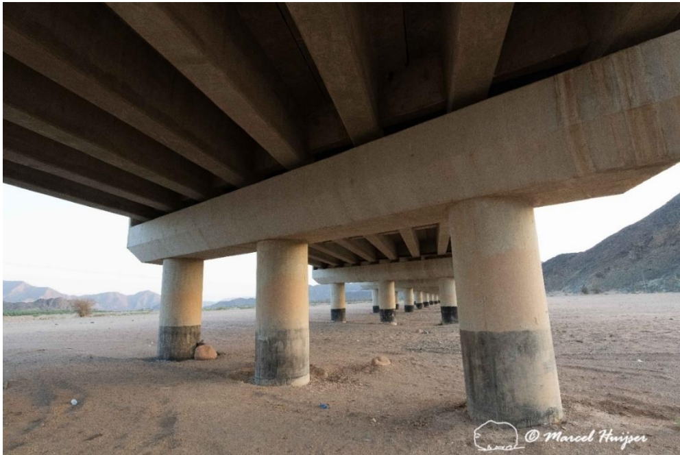
Figure 8: Supporting pillars, rather than supporting walls, allow for greater sight distance for wildlife under the bridge, Hwy 328, south of Alula near Magattyah, Medina Province, Saudi Arabia.
