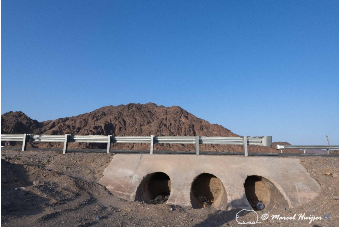
Figure 25: Plugged culvert south (downstream) of potential mitigation site for Nubian ibex ( Capra nubiana ), Hwy 328 between Masader and Jadedah, AIUla, Medina Province, Saudi Arabia.
