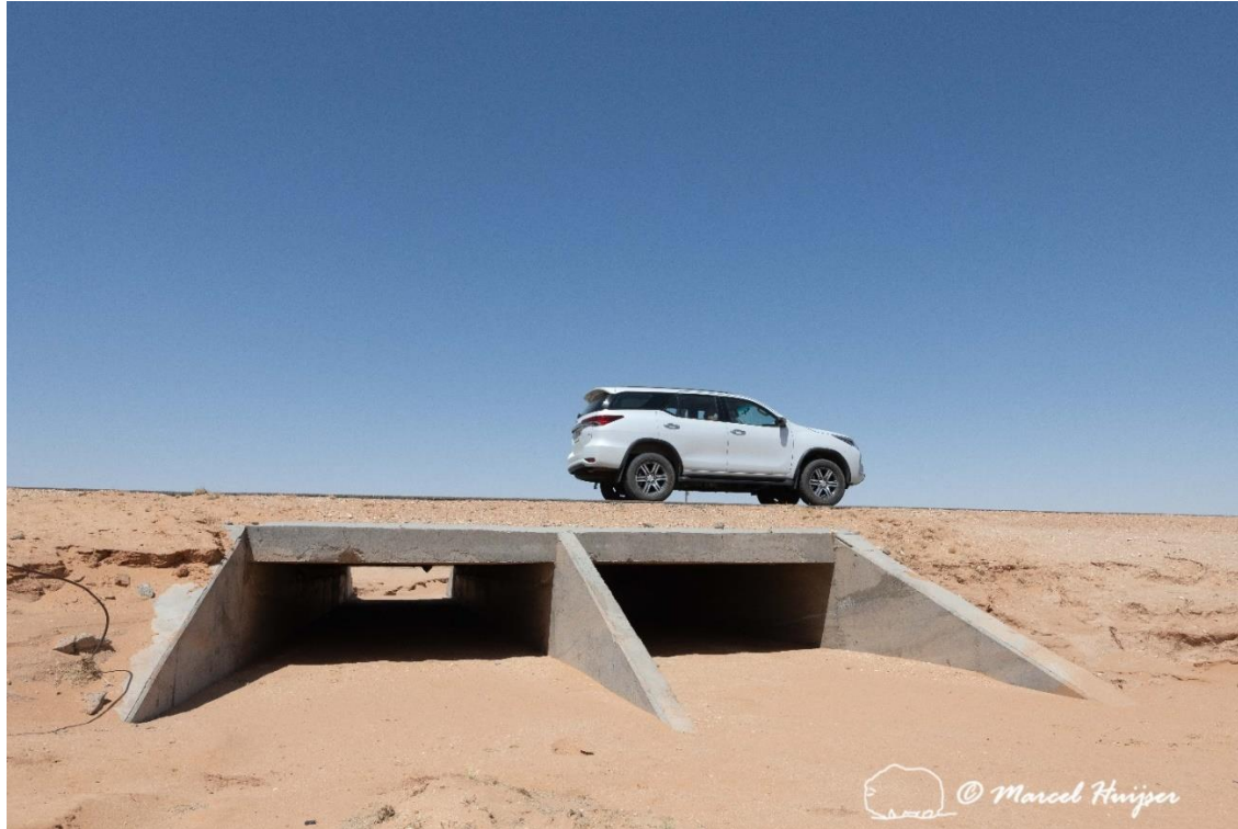
Figure 21: Inflow of a culvert to address surface flow, along Hwy 8806, AIUla, Medina Province, Saudi Arabia.
