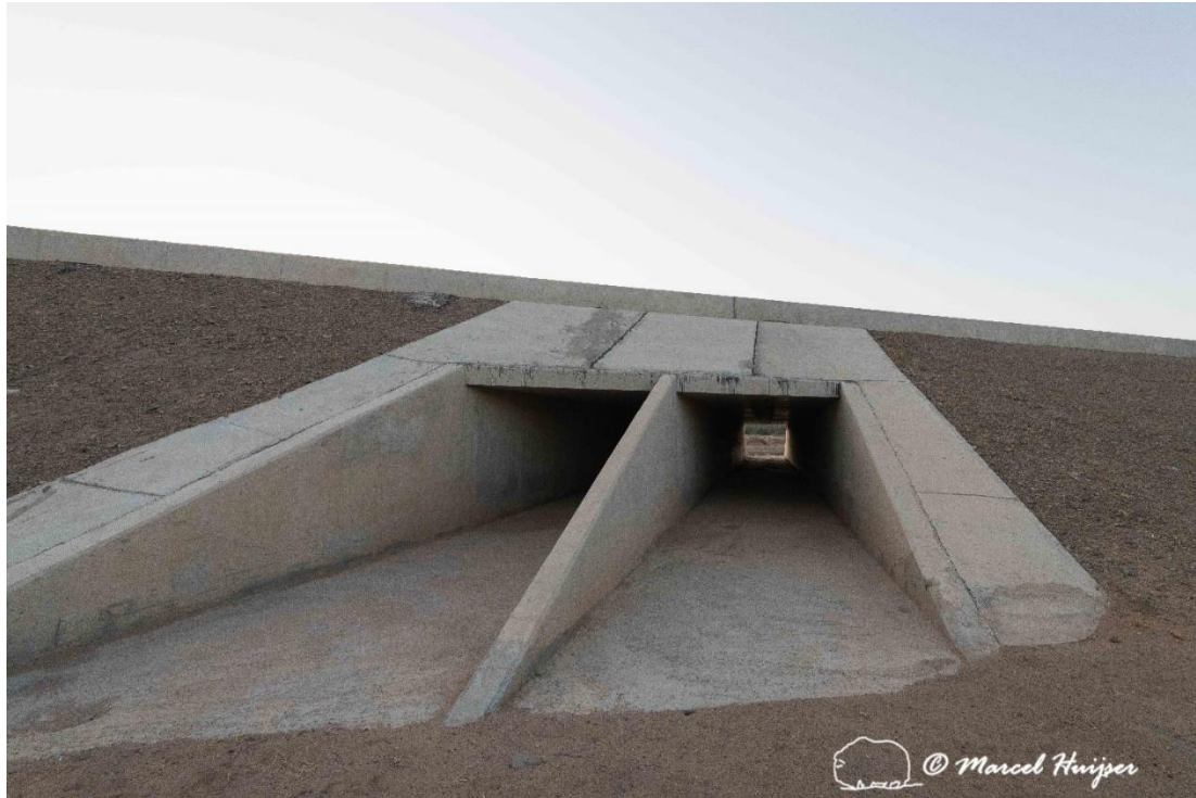
Figure 9: Double box culvert with solid dividing wall limiting sight distance for wildlife, Hwy 328, south of Alula near Magattyah, Medina Province, Saudi Arabia.
