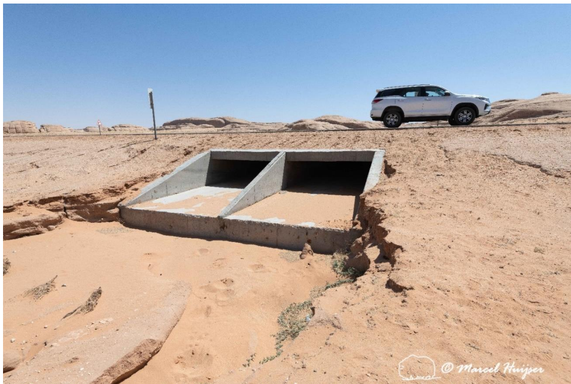
Figure 22: Erosion at the outflow of a culvert to address surface flow, along Hwy 8806, AIUla, Medina Province, Saudi Arabia. Note the drop at the concrete which forms a barrier to small animal species. The erosion also is in the process of forming a channel.
