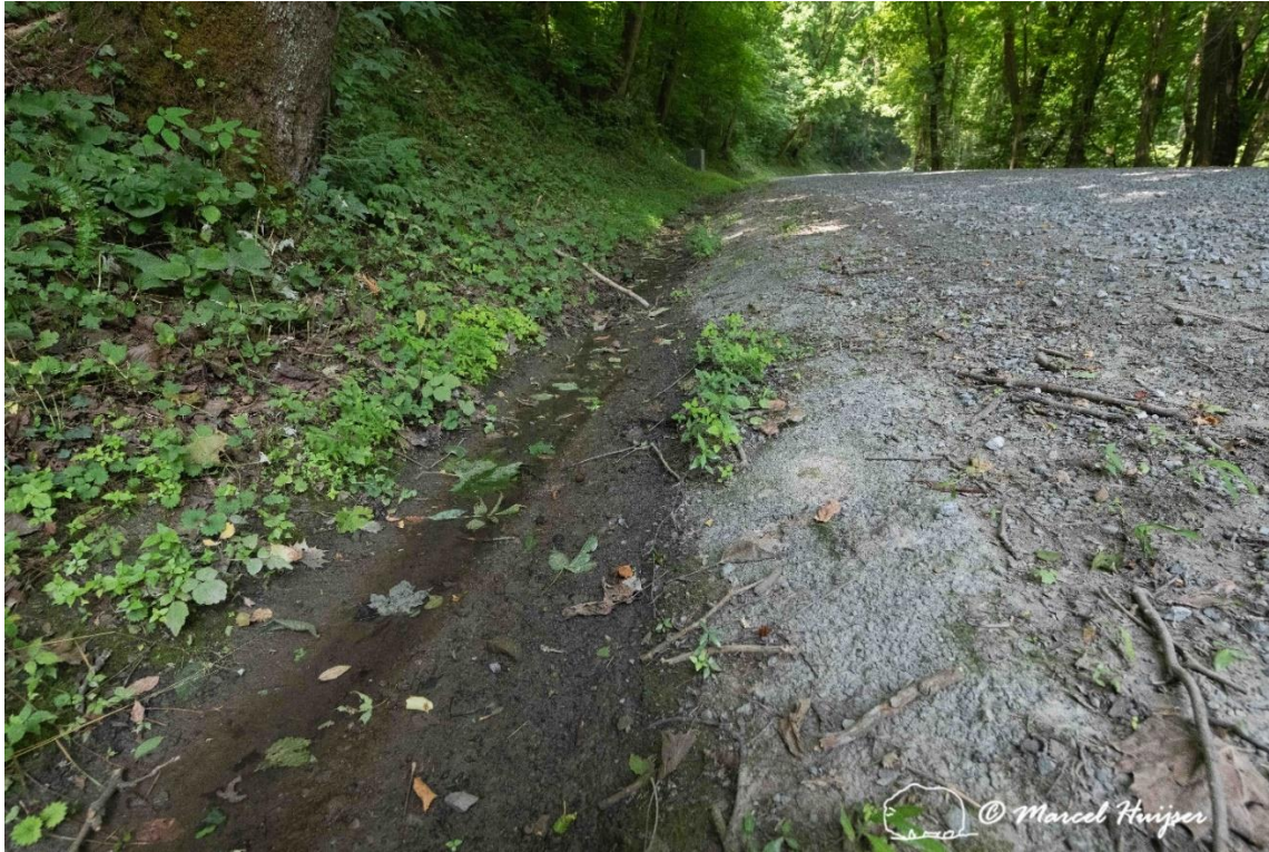
Figure 29: Inboard ditch along the gravel Glade Creek Road, New River Gorge National Park and Preserve, West Virginia.
