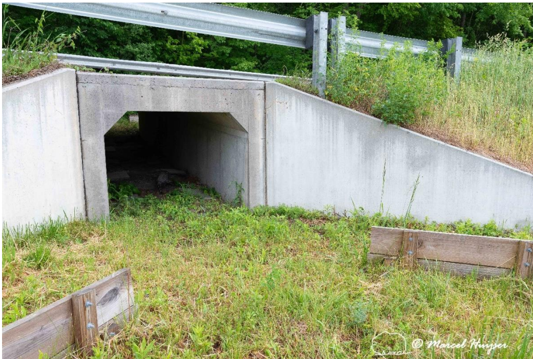
Figure 53. Underpass (culvert) for amphibians, including salamander species, Monkton-Vergennes Road Vermont USA.
