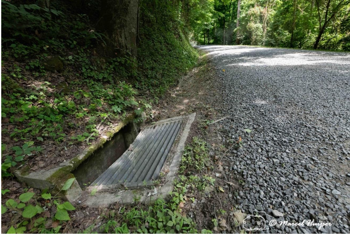
Figure 31: Storm drain along the gravel Glade Creek Road, New River Gorge National Park and Preserve, West Virginia.
